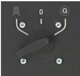
Main/generator selector switch
